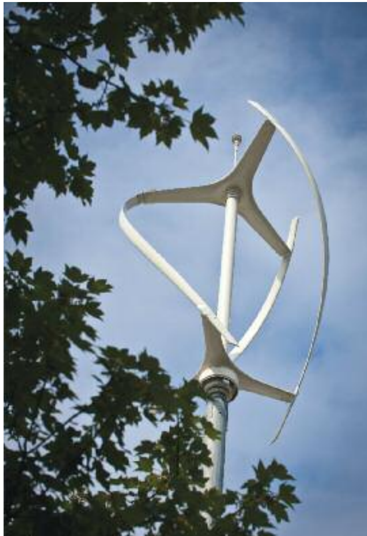
Wind turbine on Ellison Building for research into renewable sustainable energies
